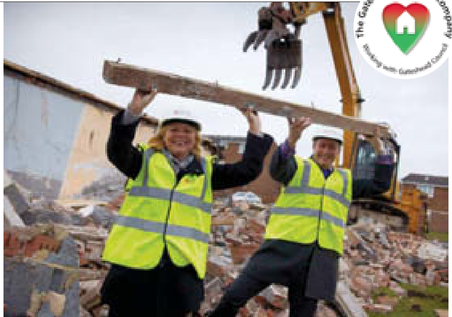
Councillor Angela Armstrong, with The Gateshead Housing Company's Acting Director of Property and Technical Services, Paul Proud, at the Portobello demolition site.
